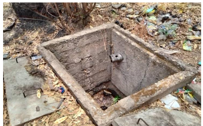
Non-functional central sewage chamber on the site
